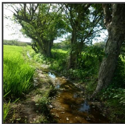
Figure 4b: Heavy growth of plants along the canals
